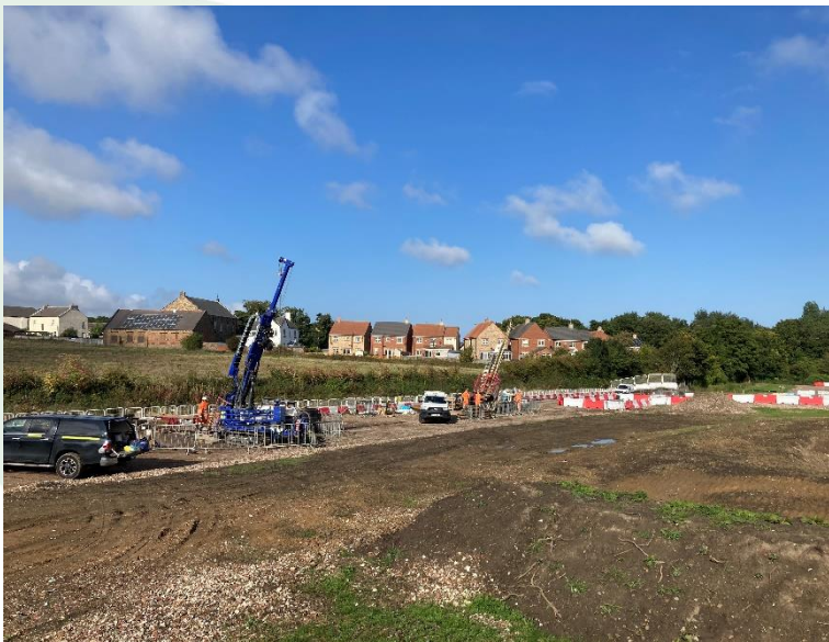
View of the mining and grouting works being undertaken at the site of Seaton Delaval station.
