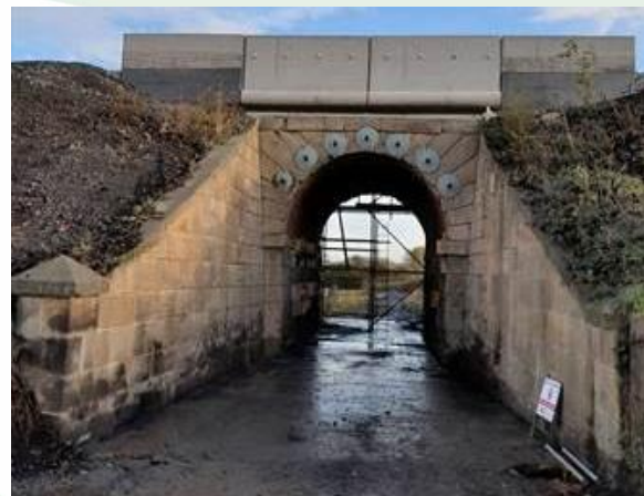
View of Underbridge 42 from the footpath, with the arch reinforcement in place.
